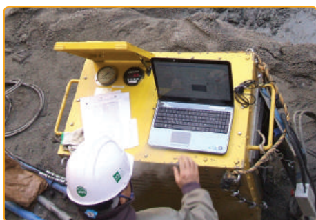
▲ Prestress Load Control Pump
