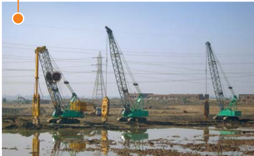
▲ New Bong Escape Hydroelectric Power Complex (PAKISTAN)
