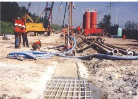
Water Intake Station, Sokcho
