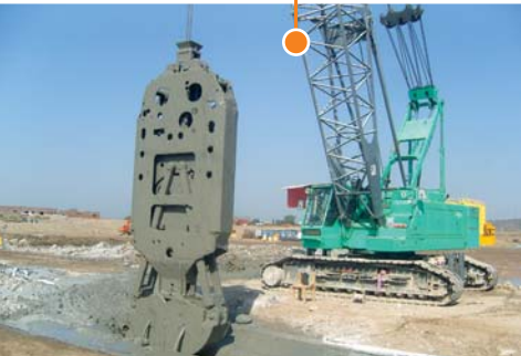
▲ New Bong Escape Hydroelectric Power Complex (PAKISTAN)
