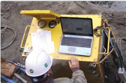
▲ Prestress Load Control Pump
